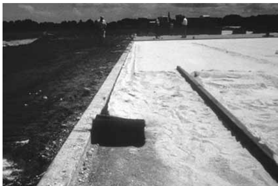
Figure 7. Woven geotextile used to contain bedding sand from migrating laterally. Visit www.icpi.org for detail drawings.
