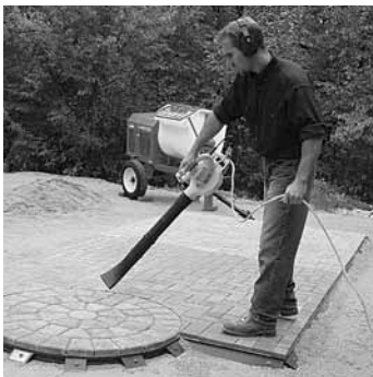
Figure 6. Whether using liquid or dry joint stabilization materials, the surface of the pavers should be cleaned with a blower or broom after the joint sand is compacted into the joints.
