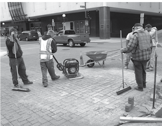
Figure 15 and 16. Reinstated pavers leave no ugly patches nor do they weaken the pavement.
